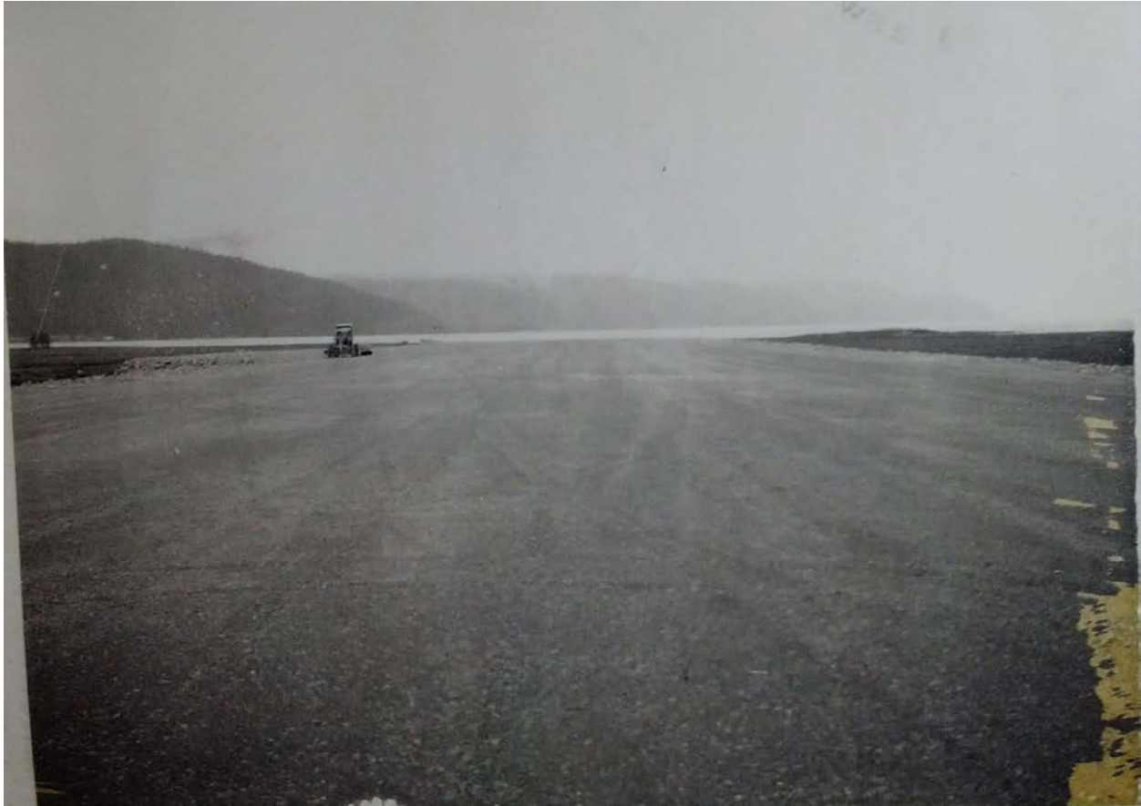
Figure 11. Overview of southern end of runway 13-31 after DOT&PF had 75% compaction from contractor in July 1966, facing southeast. Photo from DOT&PF archives.
