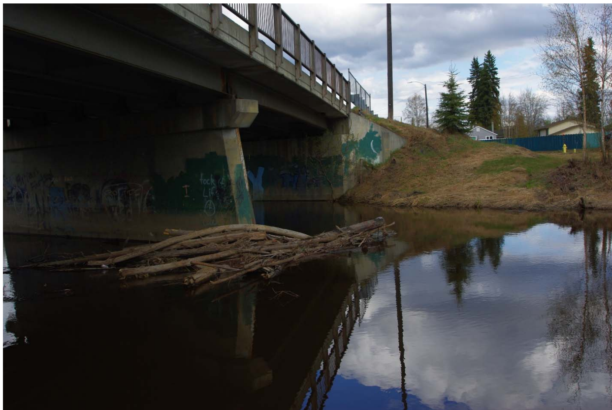
Figure 2. Center pier at the existing bridge accumulates floating logs and debris, creating the potential for increased flooding or scour of bridge foundations. The replacement bridge will be single-span, without a center pier.
