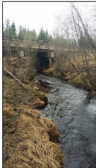
Photo 5-1 Little Goldstream Creek debris, looking downstream
