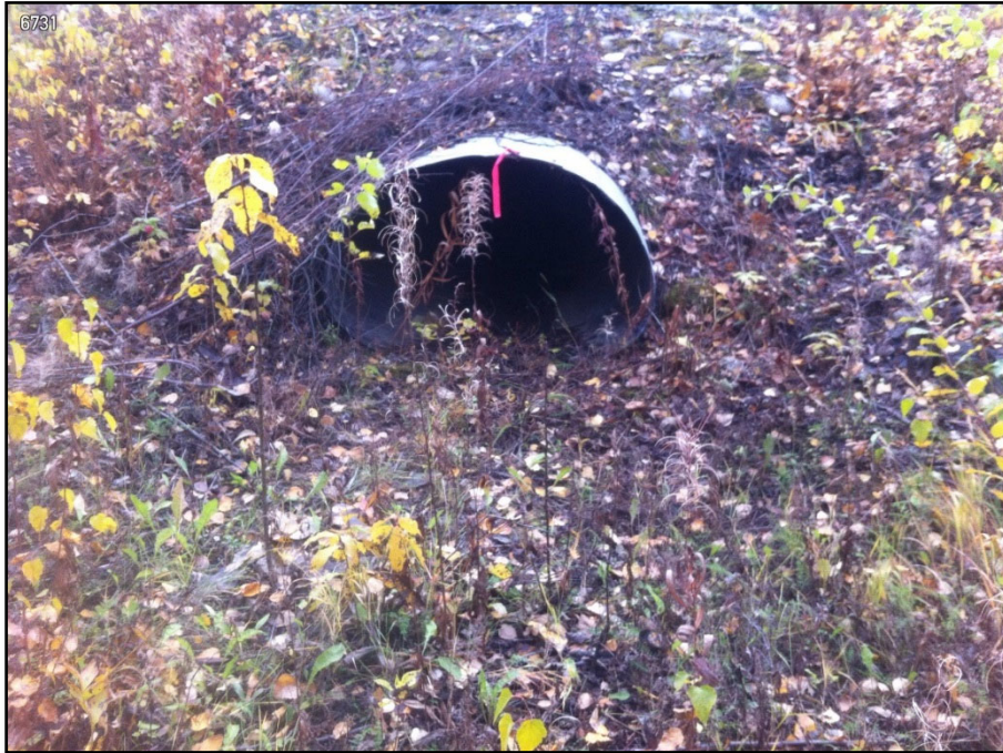
Photo 3-6 Parks Highway MP 310.6 3.2-ft H x 4.7-ft W culvert outlet, southbound side of road
