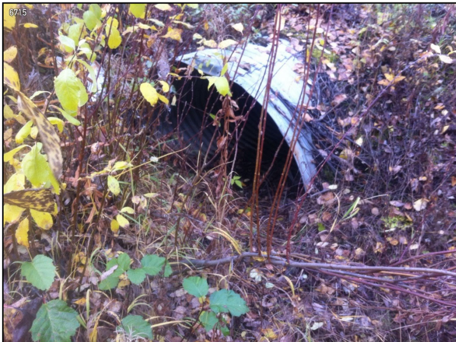
Photo 3-5 Parks Highway MP 310.6 3.2-ft H x 4.7-ft W culvert inlet, northbound side of road
