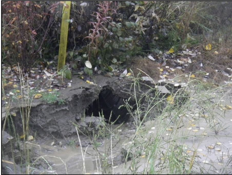
Photo 3-9 Parks Highway MP 309.6 culvert siltation
