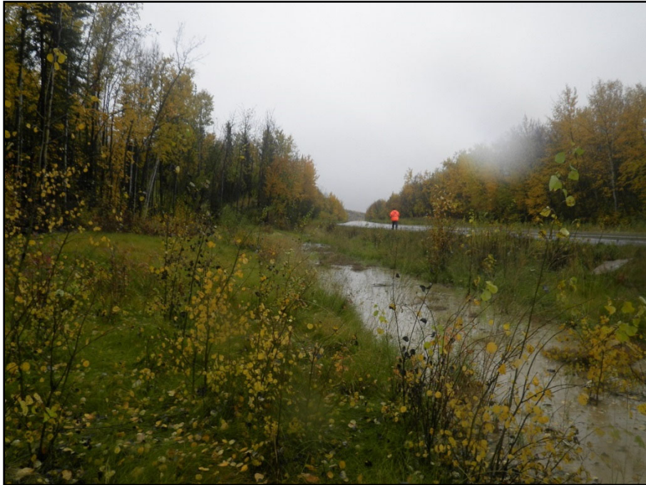
Photo 3-4 Parks Highway MP 311 drainage ditch, looking southeast from northbound side of road
