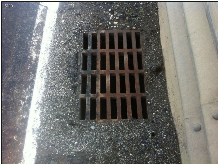
Photo 3-1 Parks Highway MP 305.4 storm drain catch basin inlet, southbound side of road
