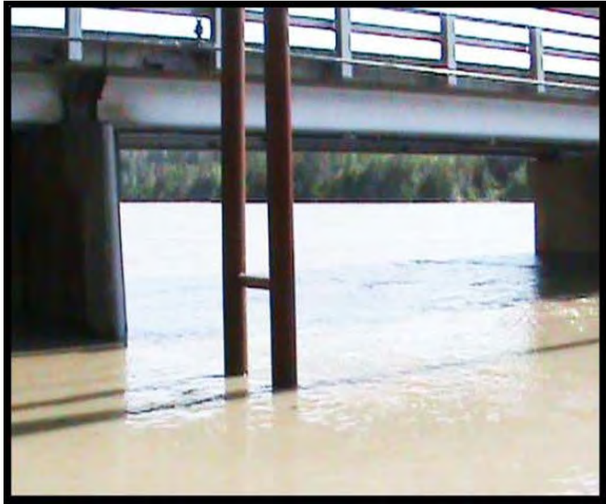
Photograph 3: Bridge Low Clearance
