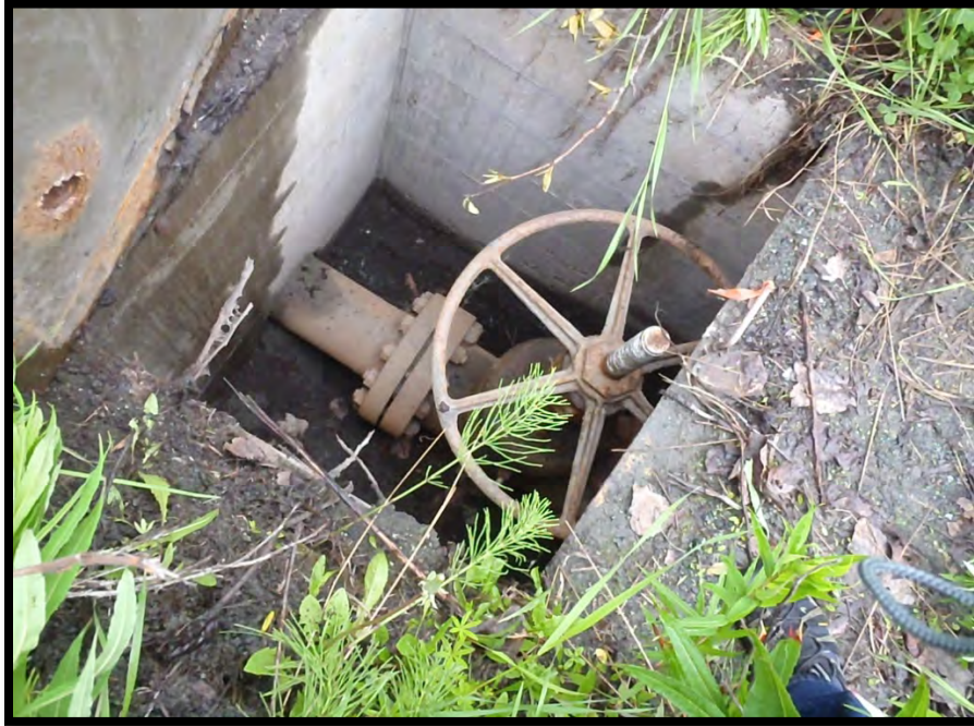
Photograph 4.10-1: Haines-Fairbanks Pipeline Gate Valve 4
