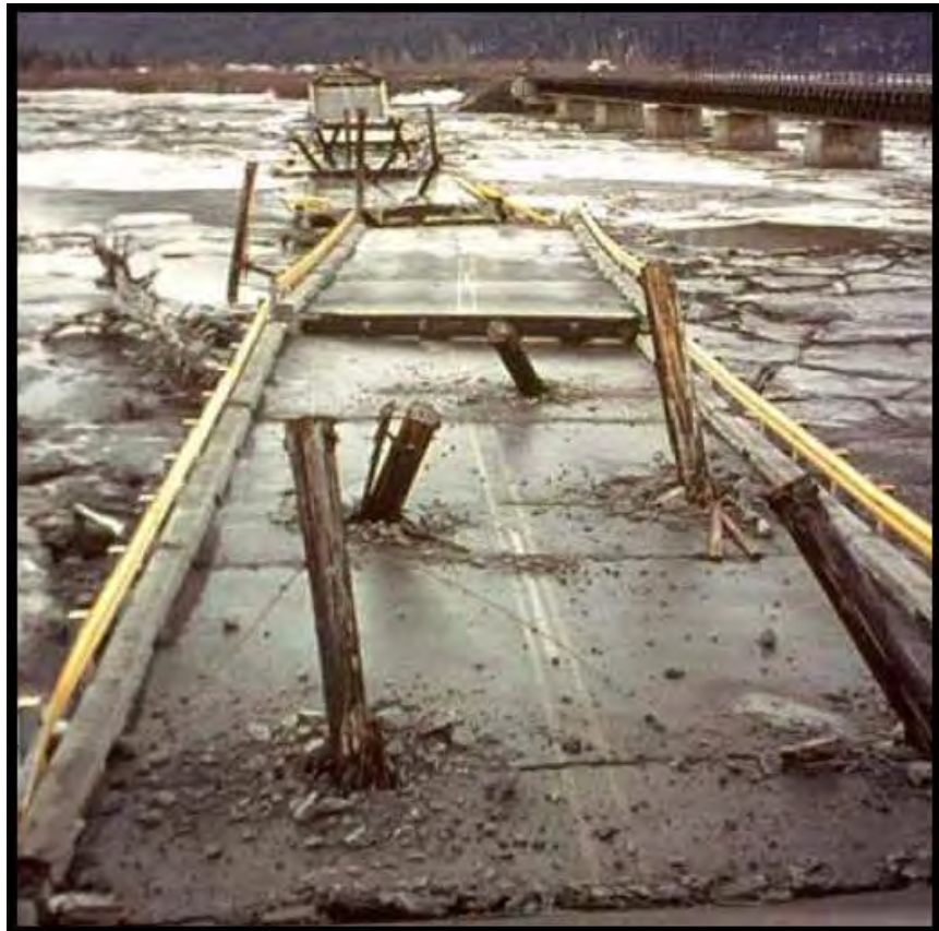
Photograph 2: Example of Bridge Damage from Earthquake
