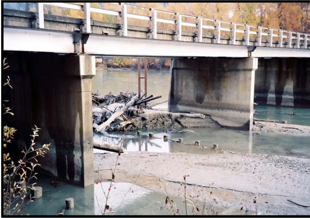
Photograph 4.12-1: Logjam Underneath Bridge
