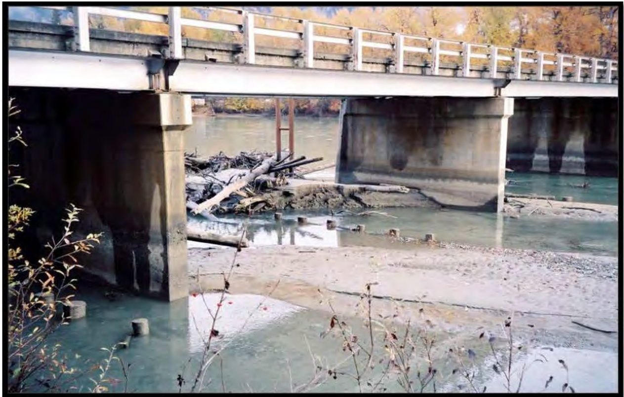
Photograph 4: Logjam Underneath Bridge
