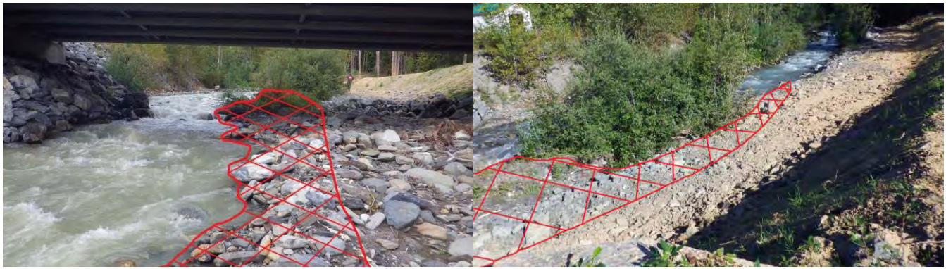
Figures 11 & 12. Left: Looking upstream from beneath the bridge at constricted section with recommended fill removal outline in red. Right: Looking upstream from the bridge with approximate recommended fill removal outline in red.
