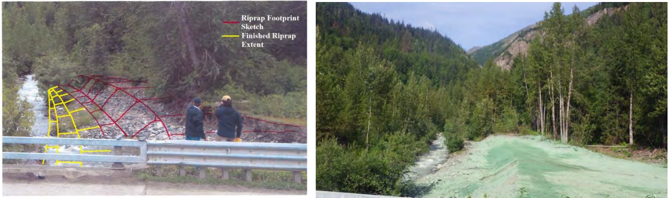
Figures 7 & 8. Left: Diagram comparing riprap plans and finished extent of riprap placed. Right: Finished bank stabilization after recent hydroseeding. Note the clump of trees in the bottom left corner of the photos gives a reference to compare the sketch and final work (August 5, 2013).
