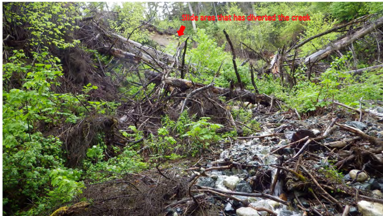
Figure 4. Looking upstream above the highway at stream no. 115-32-10250-2016-3020 headwaters and a landslide. The arrow shows where the slide occurred that diverted the creek.
