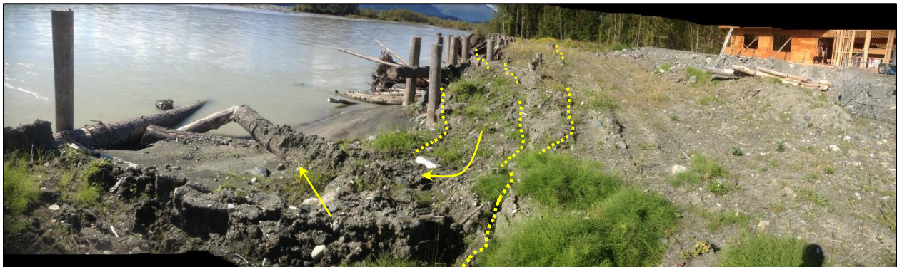
Figure 6. Wood/soil revetment structure along the Chilkat River, Klukwan, Alaska. Dashed lines indicate approximate locations of longitudinal cracking of the ground surface in the immediate area. Arrows indicate direction of bank slumping and material loss. (ADOT&PF August, 2013).
