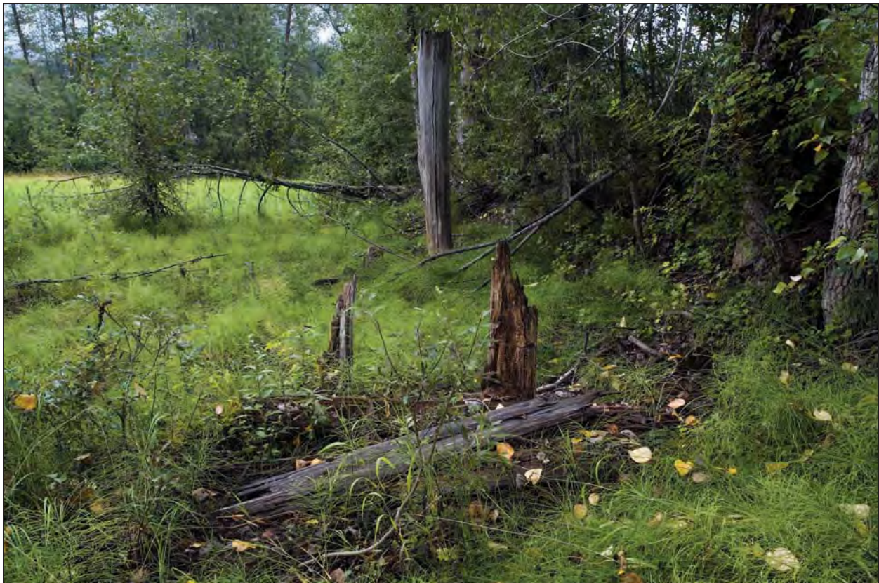
Figure H-5. Remains of timber trestle bents from the first bridge crossing at Wells (SKG-548).
