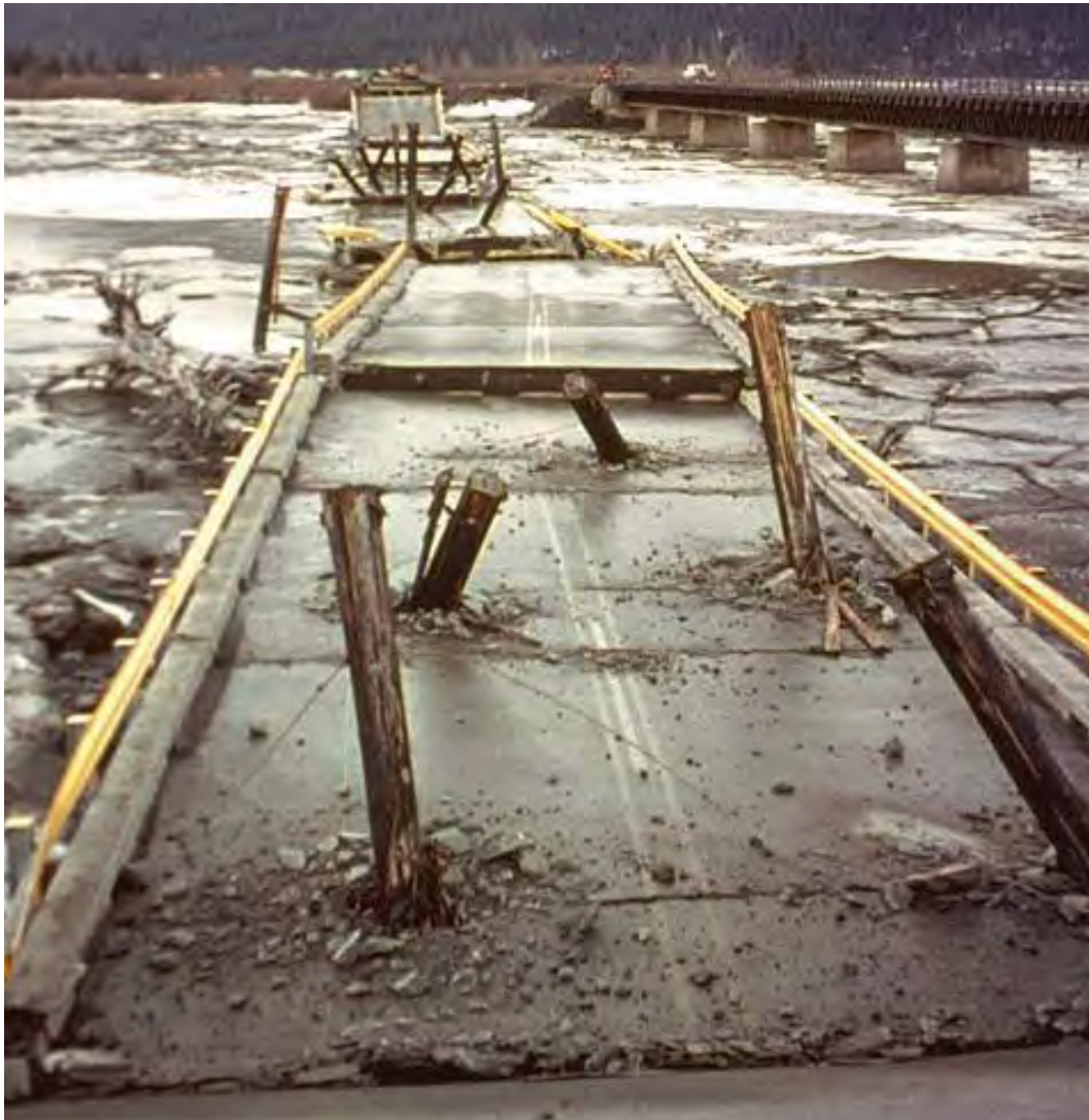
Figure 5 - Earthquake induced bridge damage (Alaska 1964)
