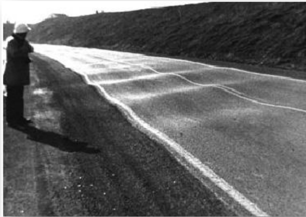
Rolling roadbed due to permafrost
