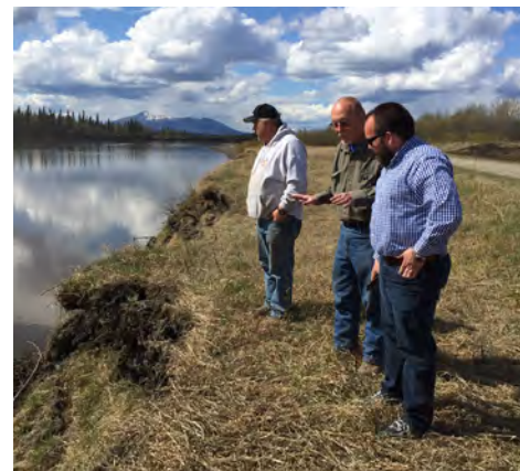
DOT&PF staff and McGrath leaders viewing erosion problems at McGrath airport
